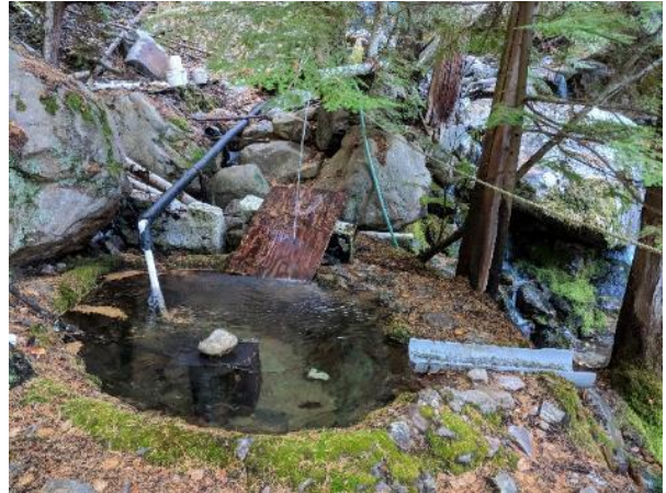
Photo 2. Water system upstream of fan
